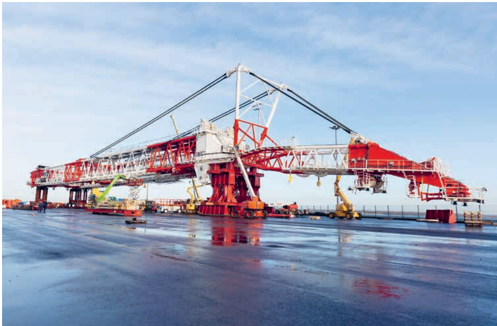
Not half bad: the boom on the HLC 295000 crane is 149 meters long. At the Liebherr site in Rostock, it is constructed directly on the Orion special-purpose vessel.
